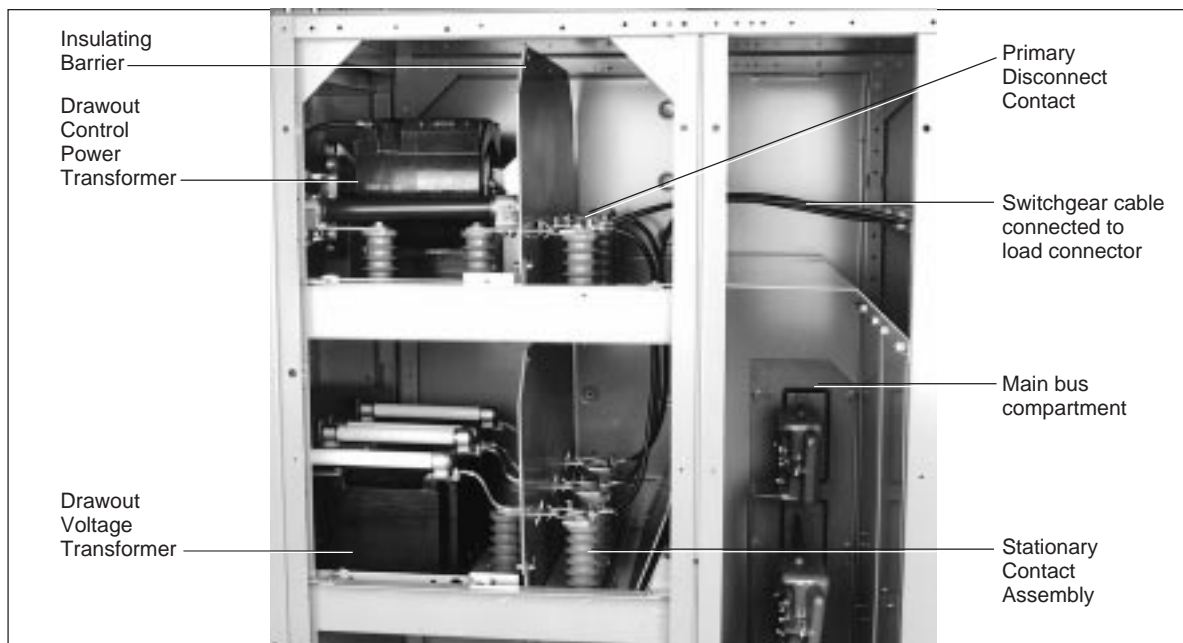
Figure 14: Drawout units in connected position
