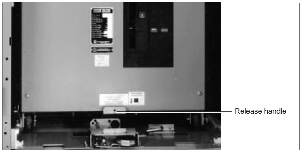
Figure 7: Circuit breaker release handle
